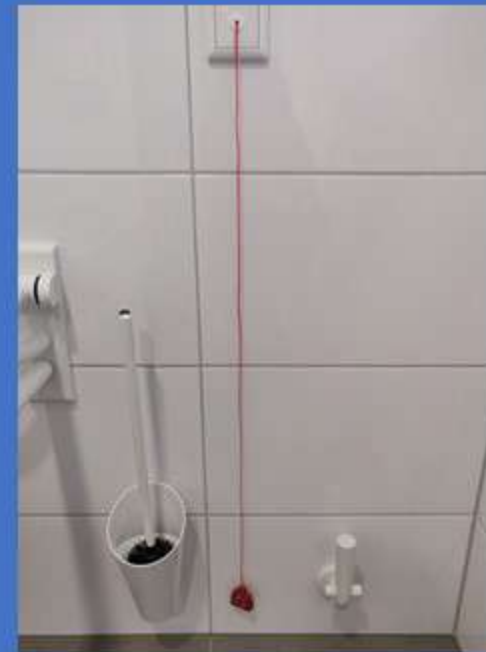
String type alarm system
