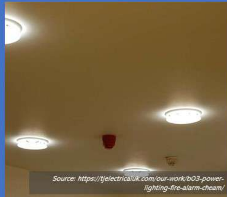
Flashing Beacon as a fire alarm system
