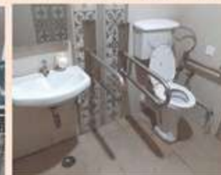
Accessible Toilet with grab-bars
