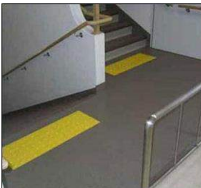
Figure 7-9: Warning blocks at landings
